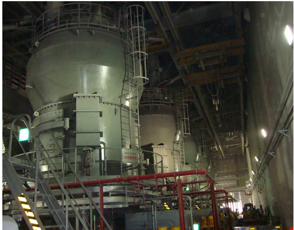
Figure 5. Physical photo of coal mill in power plant.
