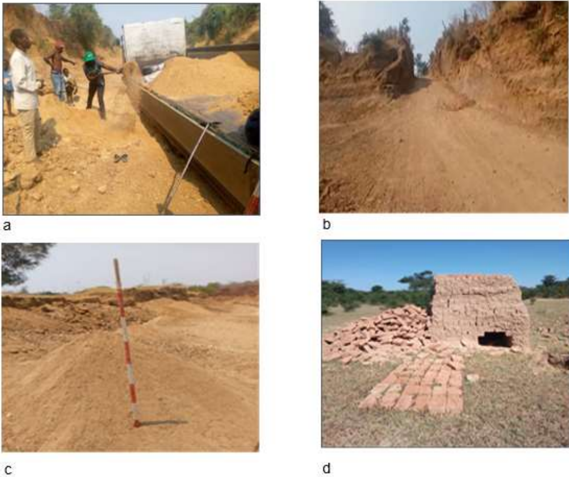
Fig. 5. Showing (a) Sand collection (b) Vehicle access roads (c) Sand cone (d) Brick moulding
