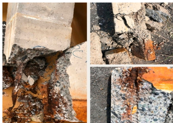
Figure 8. Corroded GPC and OPC specimens after 200 h of accelerated corrosion exposure.
