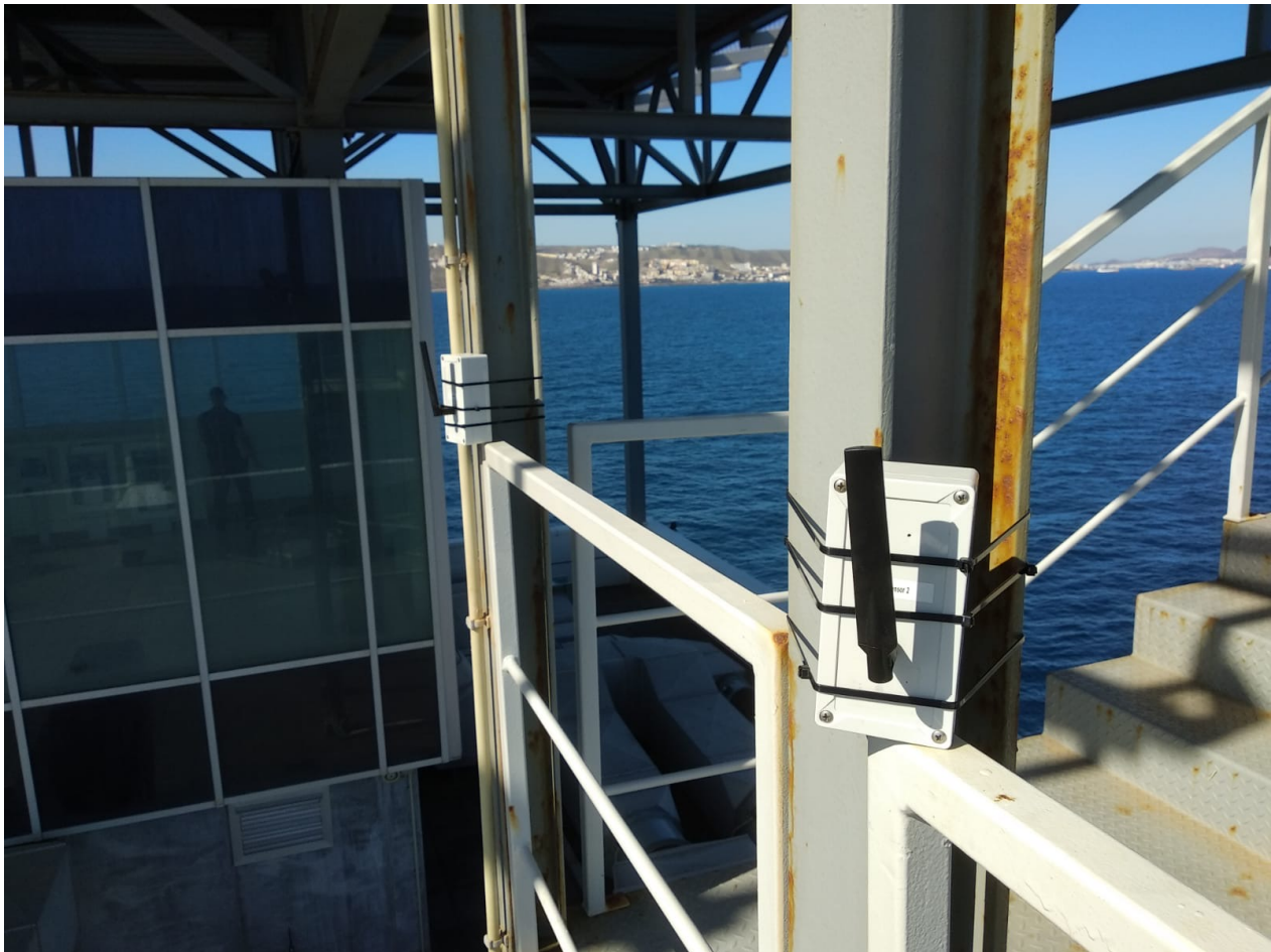
Figure 1. The sensor nodes deployed in the PLOCAN offshore platform.
