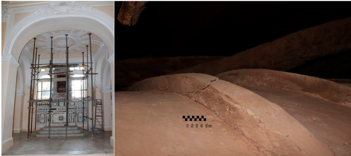
Figure 6. On the left: The intrados of the Santa Maria della Grotta's vault (Praia a Mare, South Italy). On the right: The negative bending moment in the rib, near the springer, has generated cracks parallel to the grain.
