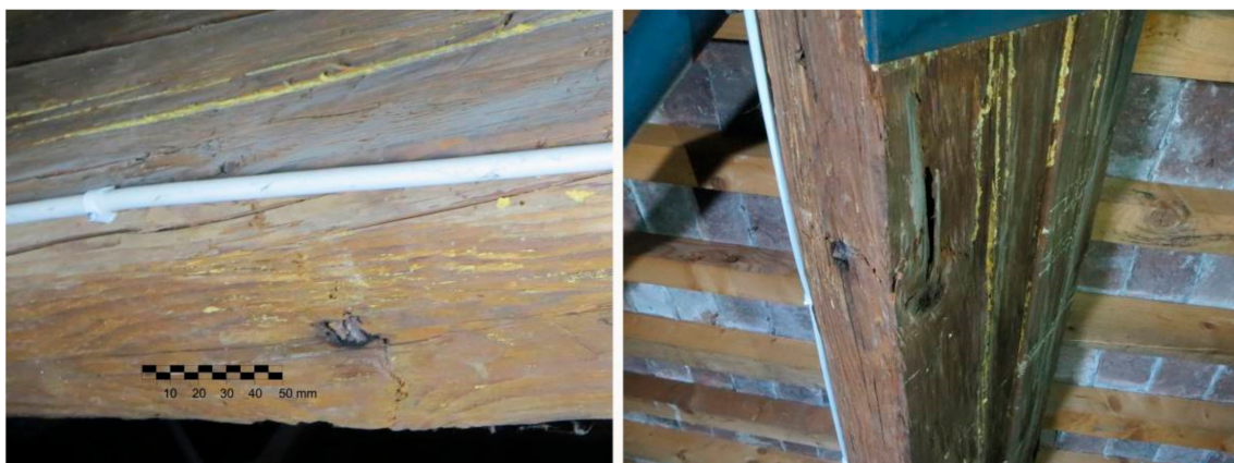
Figure 4. Roof carpentry of Palazzo Tassoni Estense in Ferrara. On the left: The crack was propitiated by the presence of a hole. On the right: The crack assumes a trend following the knot perimeter on the beam face.
