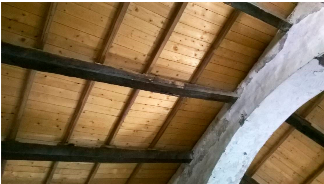
Figure 2. Cosenza (Italy), fiber delamination in a beam of the early 20th century.
